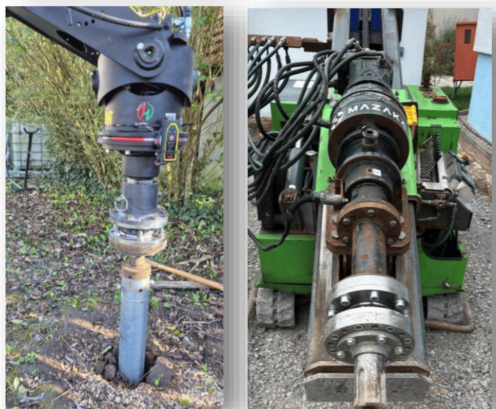
Figure 1: coreSPC 25 mounted on an excavator attachment (left) and a self-propelled hydraulic installation rig (right).
